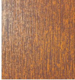
RUNNING METALLIC RUST
